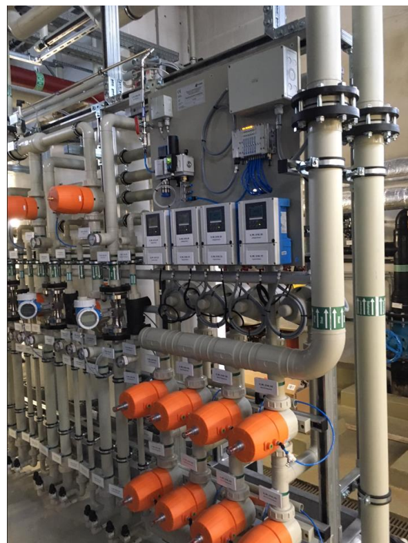
Fully automated water treatment system
