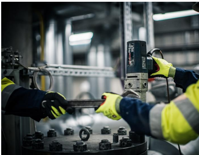
Image: Bilfinger employees install the complex plant equipment of the new district cooling center
