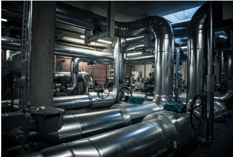
Image: Bilfinger has already supported SWM with the construction of piping for a geothermal plant
